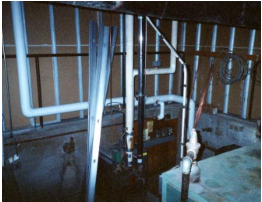
The inability to locate a serious water leak in the pipes buried in Telluride House's massive concrete foundation necessitated the relocation of hot water pipes throughout the ground floor level. This is just one of the capital projects, unanticipated and planned, slated for completion in 2001-02.
